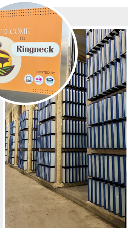
One of the filter bank rooms that filter air coming into the facility
